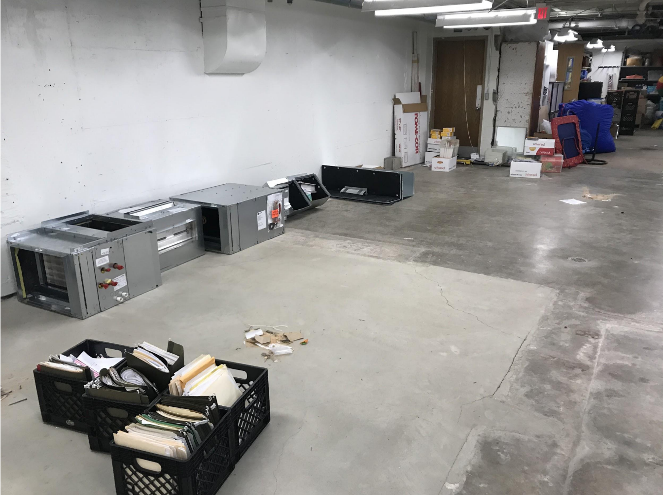
Picture below: Equipment and hardware waiting for installation that will upgrade the basement's HVAC system.
