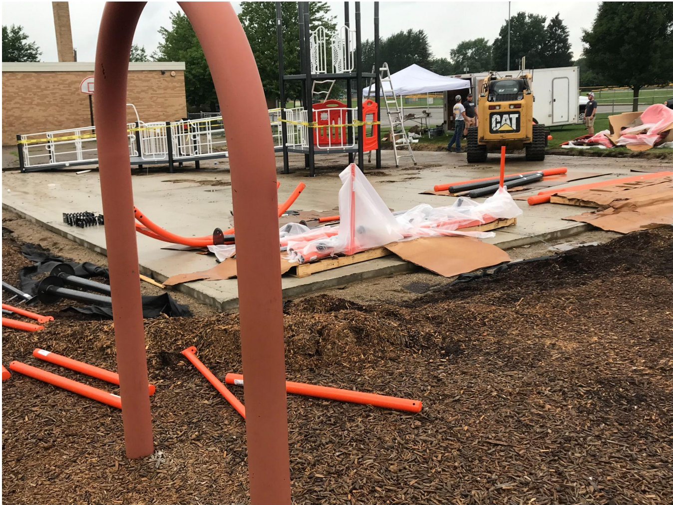
Pictured below: New equipment being installed on the playground on the East side of the school.
