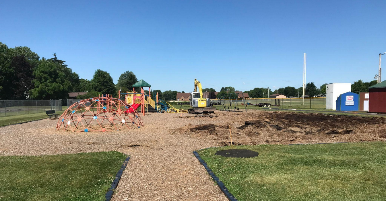
Pictured below: Removal of old equipment and readying the site to pour concrete for the tile surfacing on the playground on the West side of the school.
