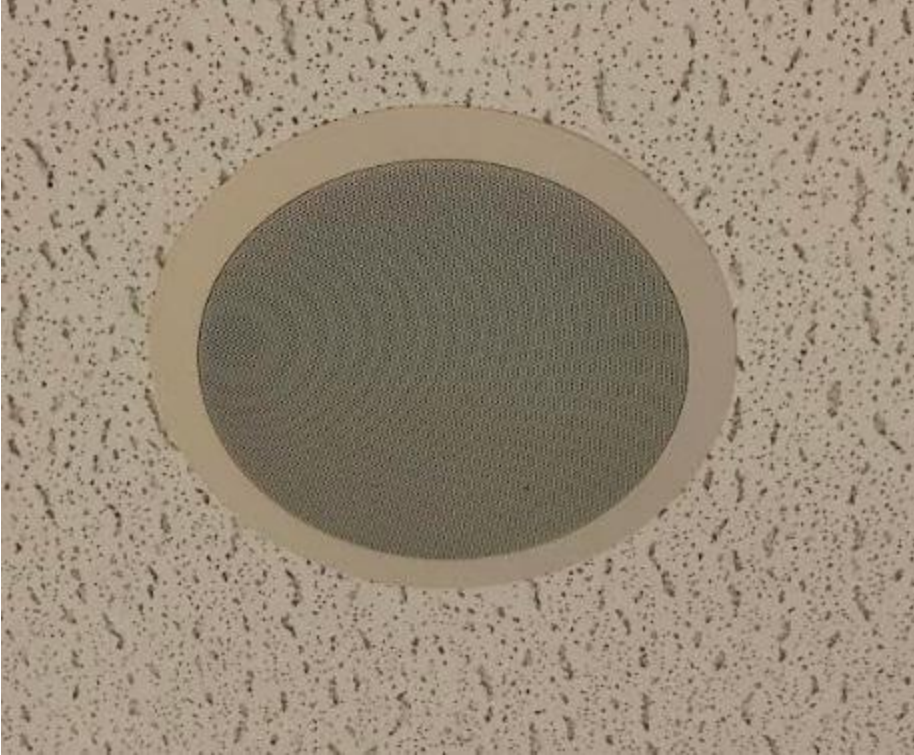
Pictured below: Ceiling speaker installed in a classroom.
