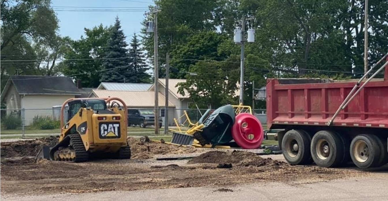
Picture below: Old playground equipment being moved, and site prep work, to make way for the new structure and equipment (from July 14, 2020).
