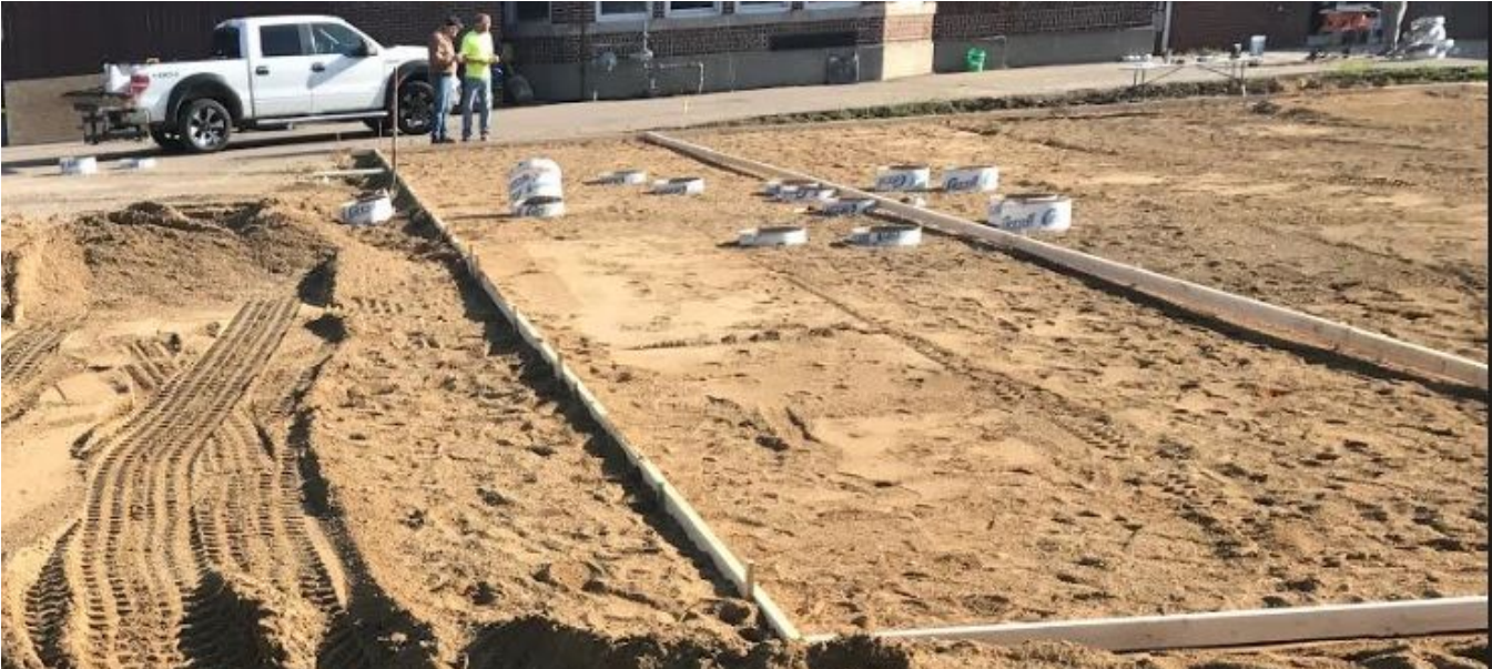
Update: 7/24/2019: The construction crew is prepping the area before pouring the concrete pad.
